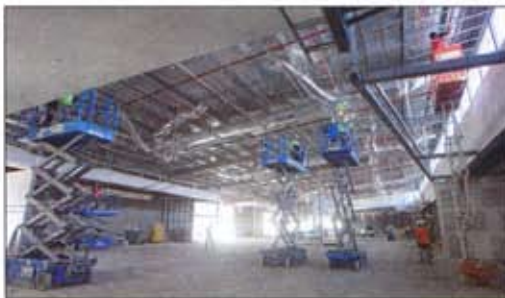
THE building, supported by 1500 tonnes of steel, has come together with the help of 150 tradesmen over the past year.
